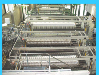
Filterpresses at Metallurgy
